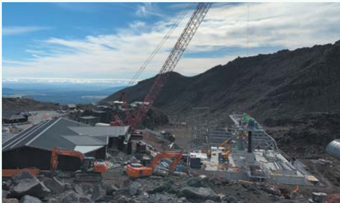
Construction underway on the drive station for the new high speed gondola at Whakapapa skifield. The project received a $10 million loan from the Provincial Growth Fund and will significantly boost the region's tourism offerings.
